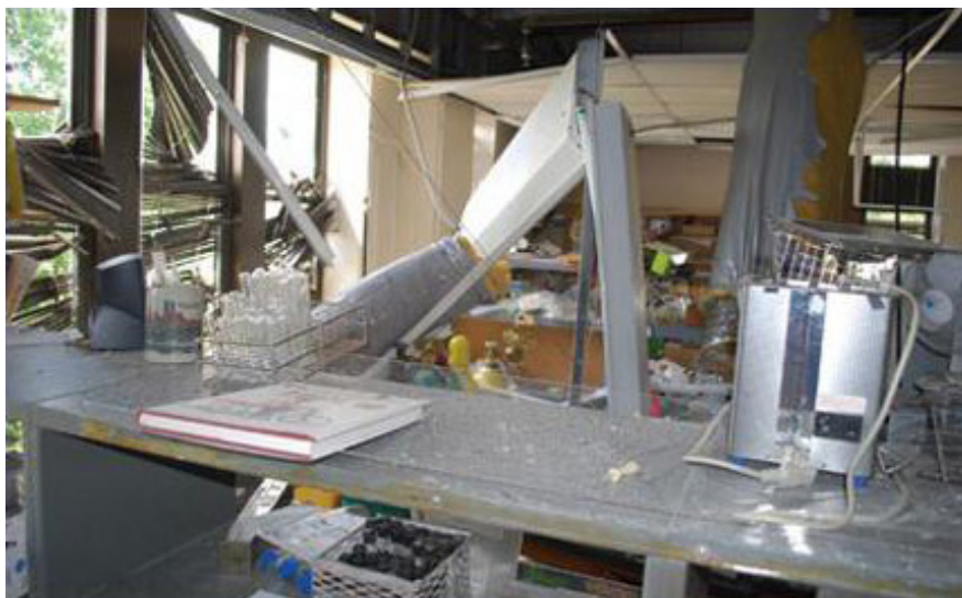
Explosion at University of Missouri in 2012. Photo courtesy C&EN
