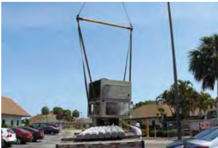
A crane is used to install the chiller unit for the cooling system used in the Scott Center.
