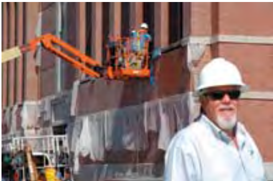
Rob Ghiotto oversees the progress on the Harris Center for Science and Engineering.
