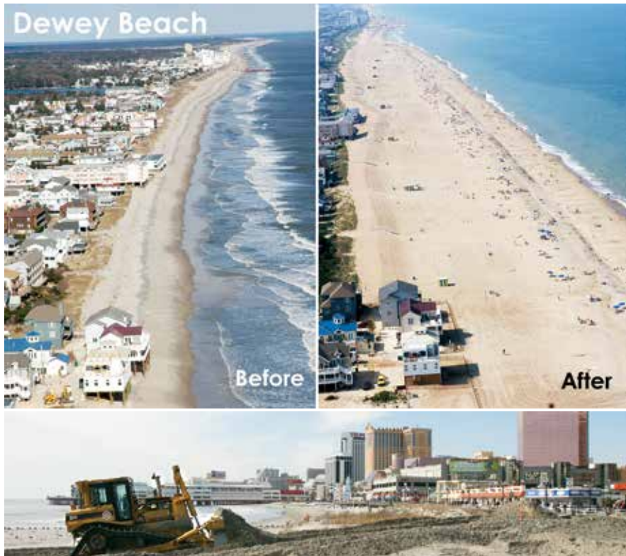
An example of the Army Corps of Engineers beachfront preservation projects: In 2005, the Corps began a federal project along the coastline from Rehoboth Beach to Dewey Beach, Del., replenishing 1,690,000 cubic yards of sand. Designed to mitigate flood and coastal storm damage, the project spans 13,500 feet of coastline.
