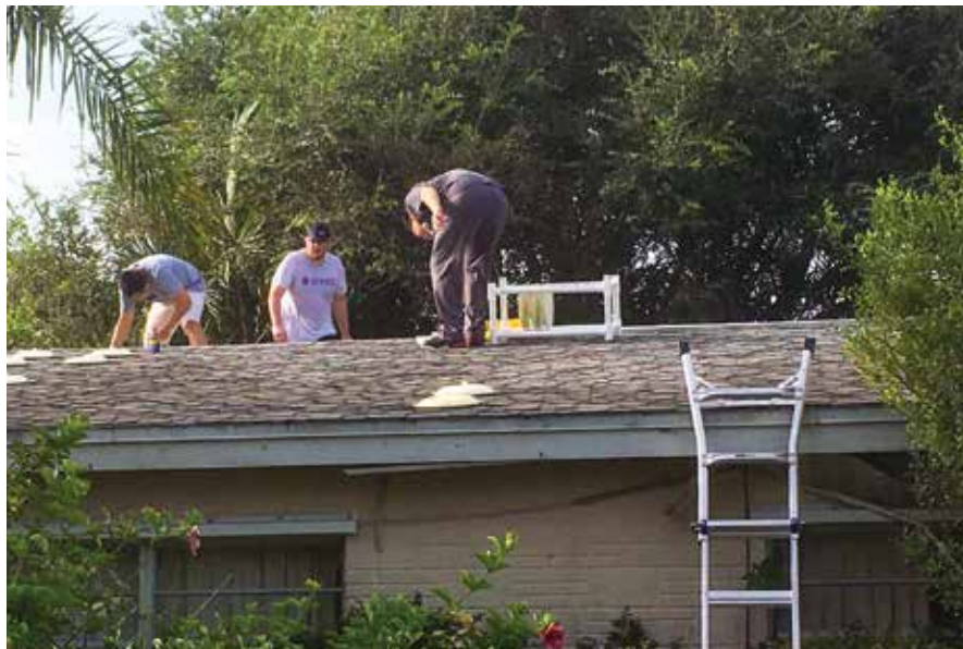
In anticipation of Hurricane Dorian, student assistants place wireless sensors on a house to measure wind profiles and provide data that could play a role in creating stronger future buildings.
